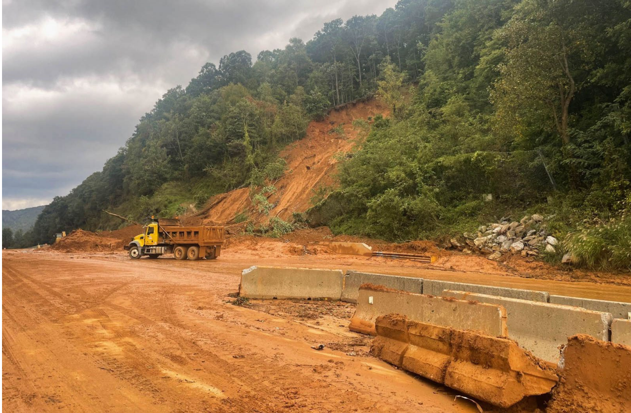
Figure 10: Aftermath of Helene-Triggered Mudslide, September 28, 2024. Credit: NCDOT
