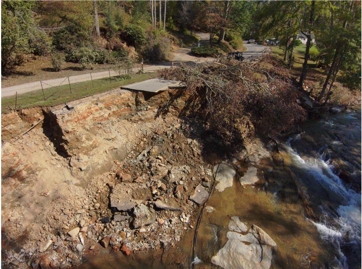
Figure 7: Bank and Road Erosion, NC Route 9, Buncombe County, NC. October 8, 2024. Credit: NCDOT
