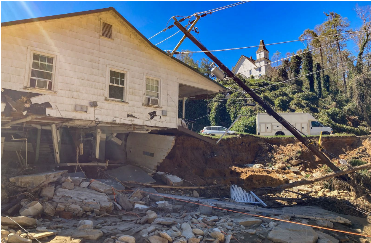
Figure 6: Housing Foundation Damage, US Route 64, Bat Cave, NC. October 10, 2025.
