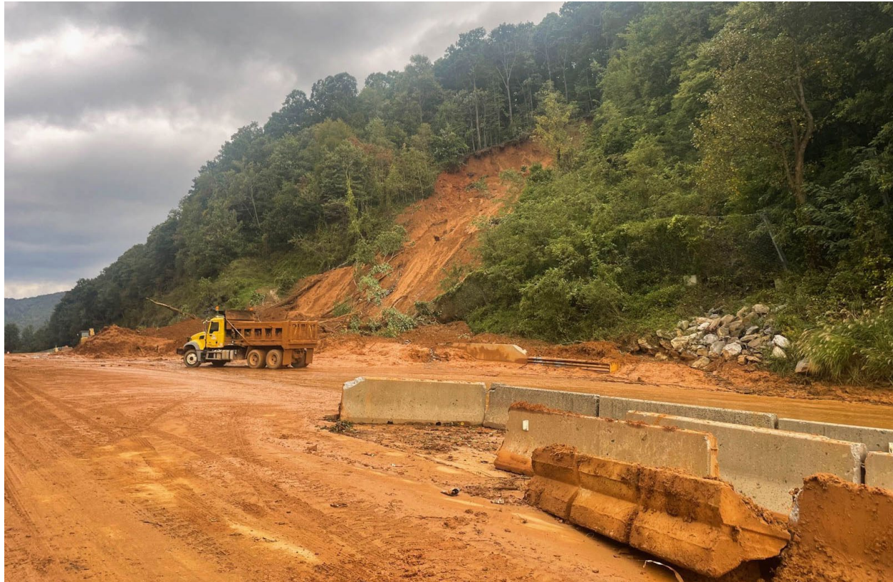
Figure 10: Aftermath of Helene-Triggered Mudslide, September 28, 2024. Credit: NCDOT
