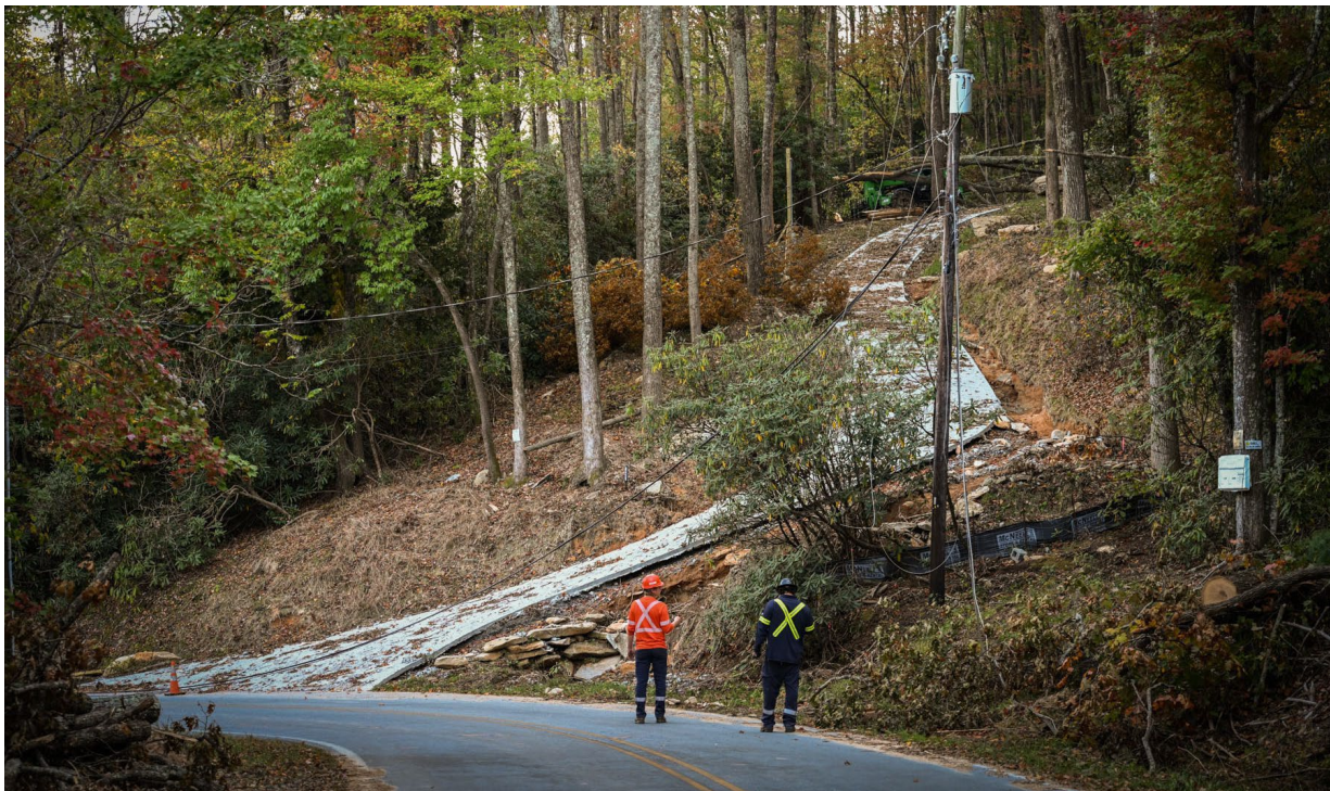
Figure 8: Photo of Damaged Private Access Road, Henderson County, October 9, 2024. Credit: NCDOT
