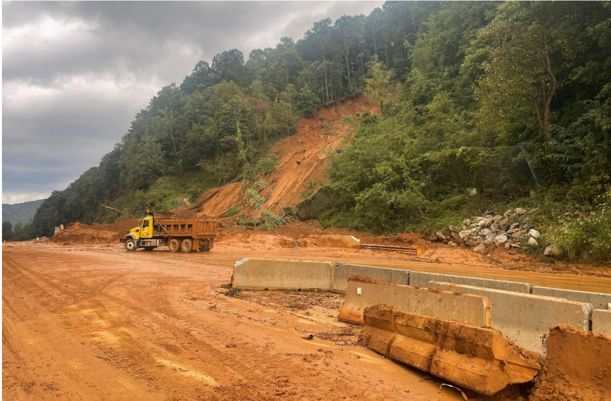
Figure 10: Aftermath of Helene-Triggered Mudslide, September 28, 2024. Credit: NCDOT
