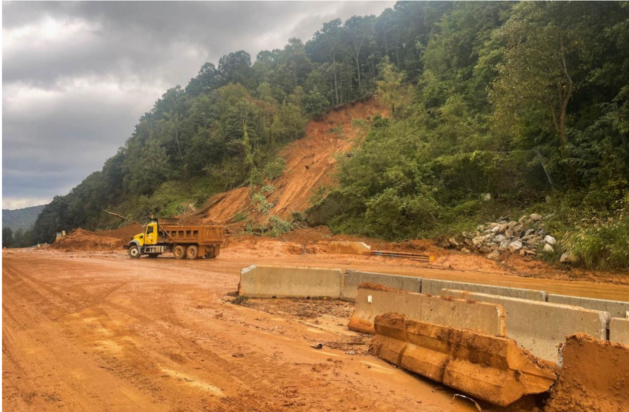
Figure 10: Aftermath of Helene-Triggered Mudslide, September 28, 2024 (Credit: NCDOT)
